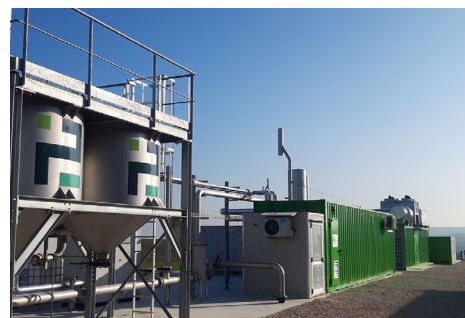
Prodeval's facility in Italy | Biogas upgrading solution
