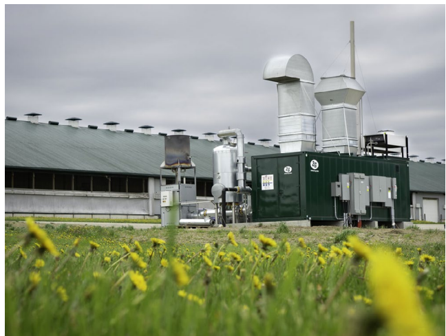
Biogas cogeneration units increase the efficiency of biomethane production Source: 2G Energy AG
